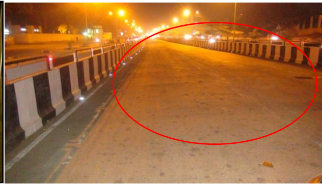
Near MES pump house
