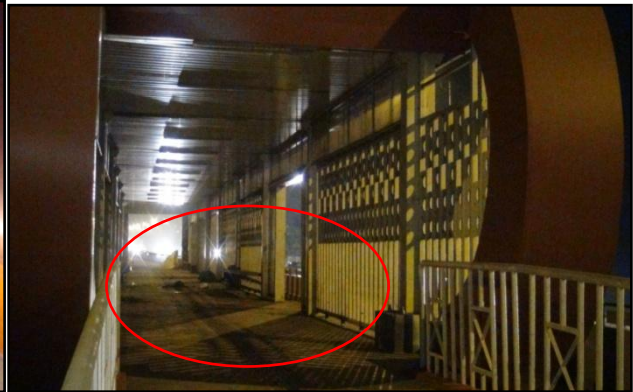
Near MES pump house
