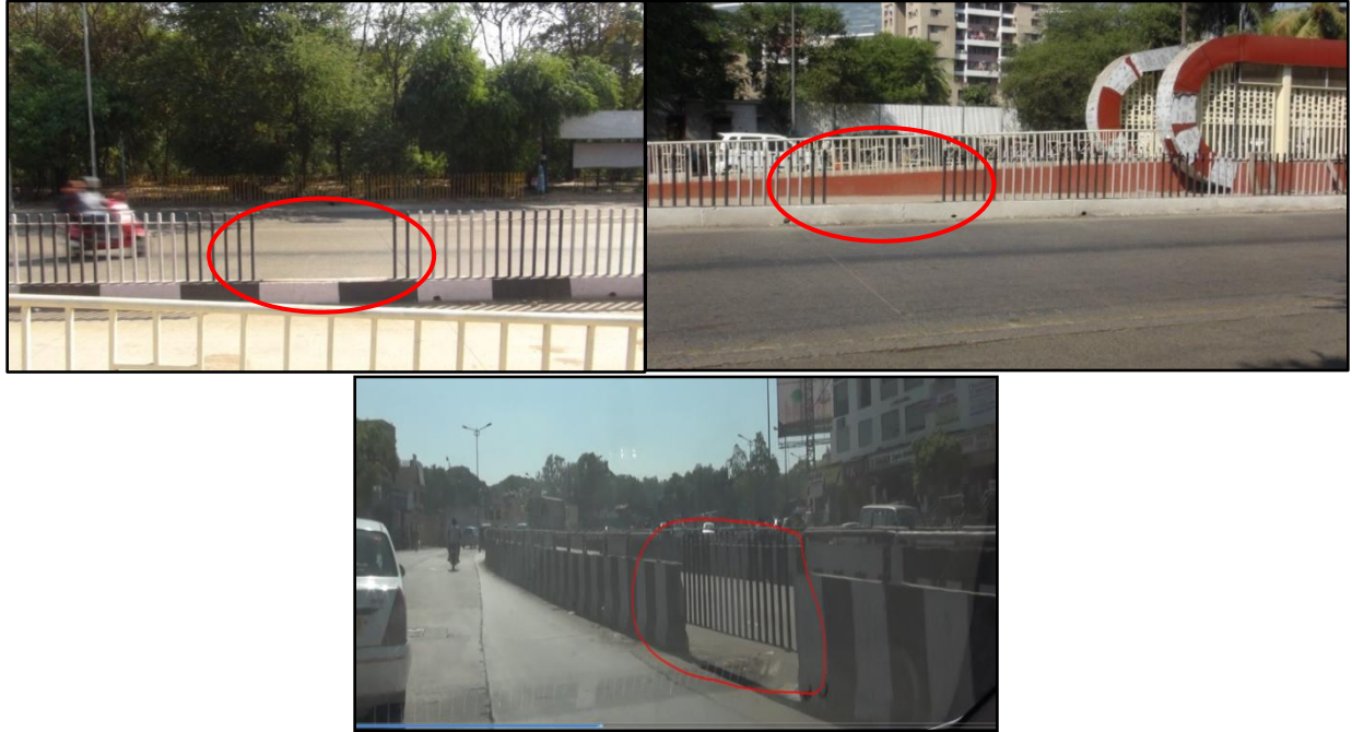
Observation 51: Inside facilities of bus station near Prince Regent is incomplete and presence of median is obstructing the BRTS foot path
